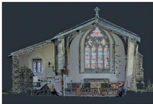
Figure 32: 3D Laser Scan Data, showing leaning Chancel Wall.
