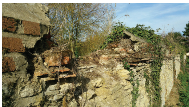
Figure 7: Damage to eastern precinct wall, Newnham Priory, Bedford
